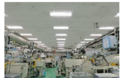
LED lighting in Yamagata Casio's plant
