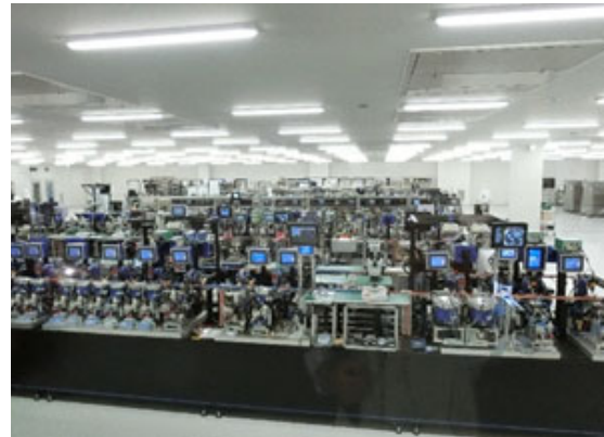
Clean room with latest air-conditioning system
