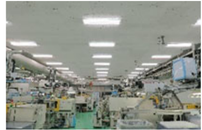
LED lighting in Yamagata Casio's plant
